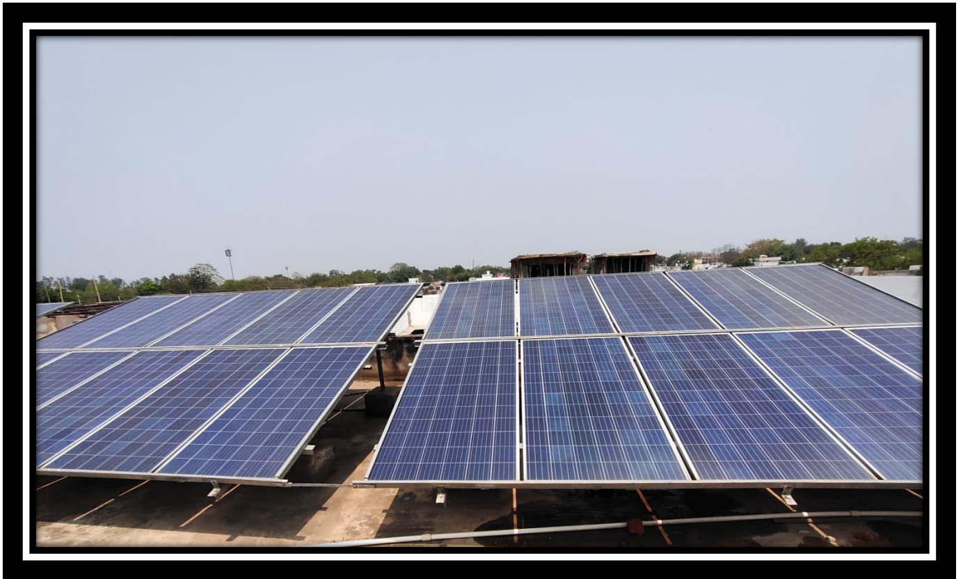
Solar Panel Equipment @ A.P.S.G.M.N.S. GOVT PG COLLEGE KAWARDHA
